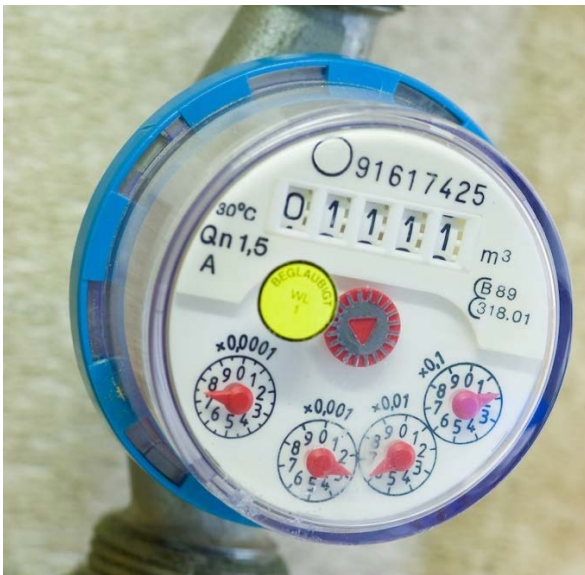
Analog Utility Meter
